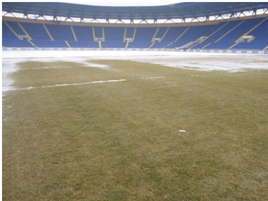
Poorly performing undersoil heating system failing to keep the surface uniformly free of frost and snow.
