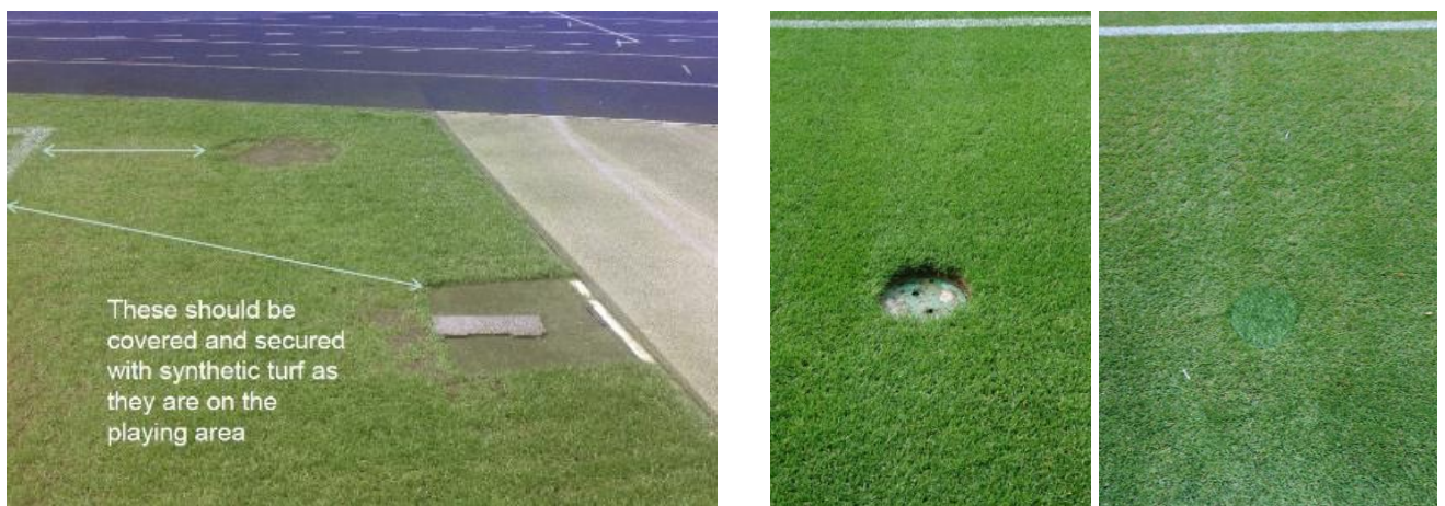
Fig. 28. Access and service boxes within the safety zone around the field of play.
